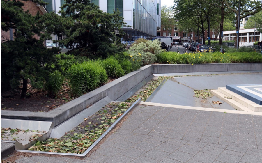
Figure 14 – Drainage channels need to be cleaned of leaves and litter or else they will clog, leading to flooding (2023).
