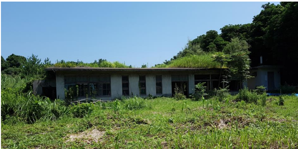
Figure 10 – Shinjima’s abandoned elementary school (photo by Henry Johnson, 2016), which was demolished in 2020.
