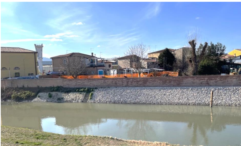
Figure 4 - Embankment blocking access to the historical Cobelli shipyard (author's photo, 2023).
