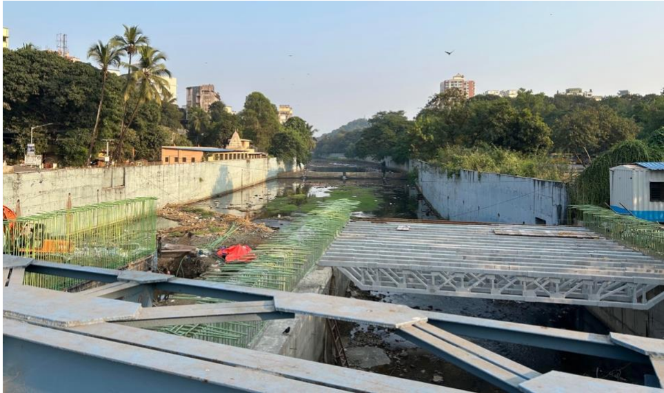
Figure 9 - Widening the existing bridge and increase in the elevated level of the bridge as a measure of flood mitigation strategy by the governing authorities (photo: Vikram Pawar, 2023).
