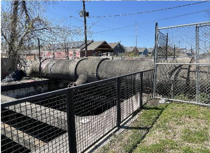
Figures 14a and 14b - Storm run-off canal and pumping station (photos by Mallum, 2022).
