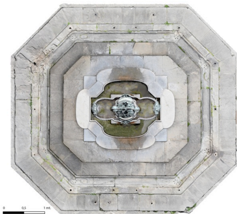
Figure 8 – Orthographic plan view of the digital 3D model of the eastern fountain in Florence.
